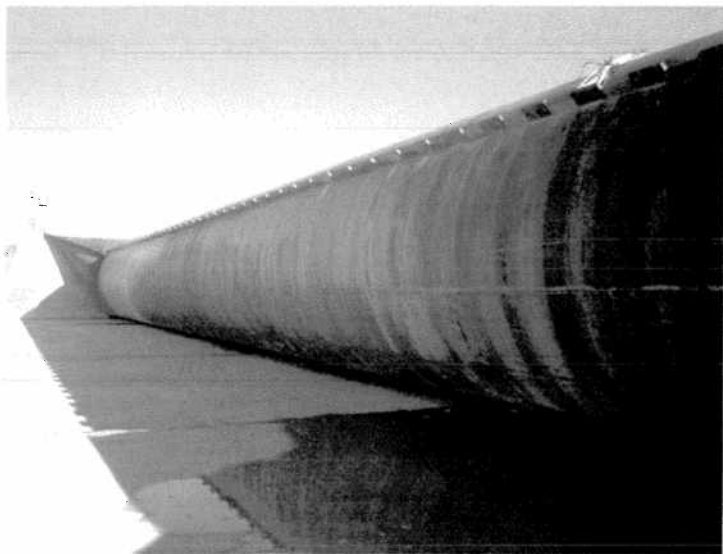
PHOTO NUMBER: 17 PHOTO DIRECTION: North DESCRIPTION: Along the downstream side of bladder #1. Bladder #1 is slightly lower than the other three and thus acts as an emergency spillway.
