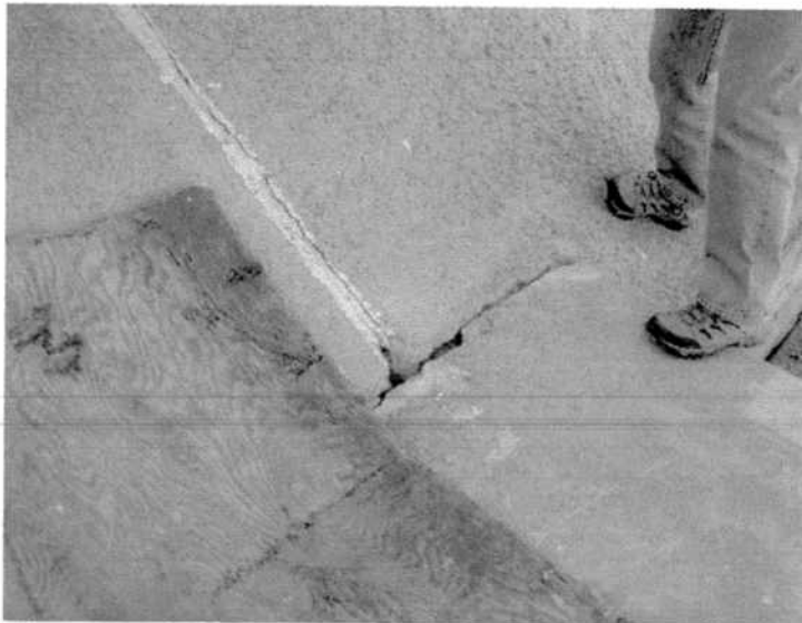
PHOTO NUMBER: 18 PHOTO DIRECTION: Down DESCRIPTION: Close-up view of cracks at the contact between the left abutment and the concrete apron. 2.5-inches long x 1-inch wide x 1/2-inch deep: Repair – seal.
