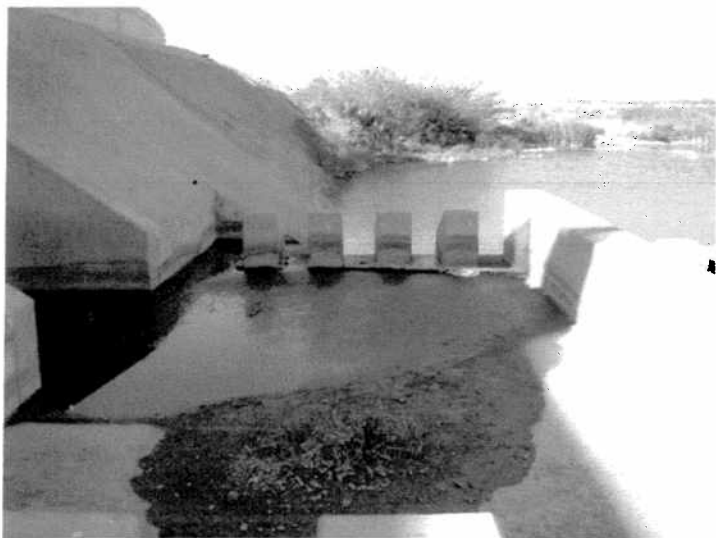
PHOTO NUMBER: 19 PHOTO DIRECTION: West DESCRIPTION: Toward downstream as seen from the foundation slab below bladder #1.
