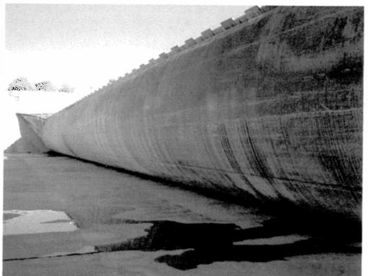
PHOTO NUMBER: 12 PHOTO DIRECTION: North DESCRIPTION: Along the downstream side of bladder #1.
