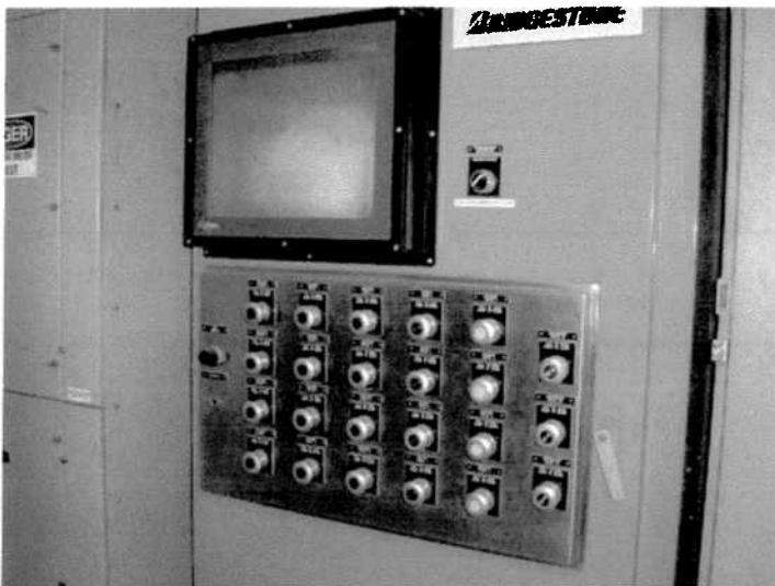
PHOTO NUMBER: 3 PHOTO DIRECTION: North DESCRIPTION: View of the PLC panel located inside of the control building above the right abutment of the dam.
